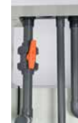
Fixed pipework made of PVC-U
